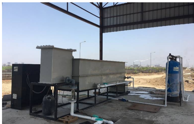
Name of Client: Merino Industries Ltd Location: Dahej, Dist. Bharuch Capacity of Plant: 60 KLD STP Status: Active / Running
