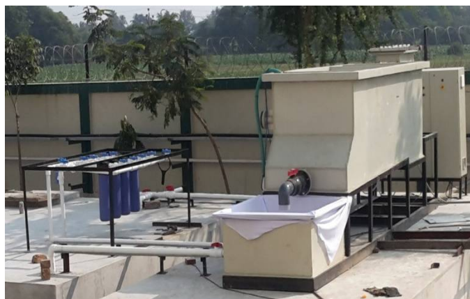
Name of Client: Standard Pesticide Pvt Ltd Location: Moxi, Dist. Vadodara Capacity of Plant: 60 KLD STP
