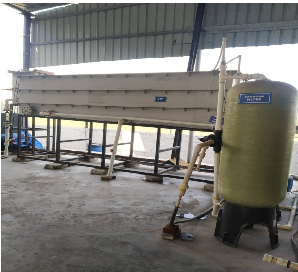
Name of Client: Global Gourmet Pvt Ltd Location: Dist. Vadodara Capacity of Plant: 100 KLD STP Status : Active / Running
