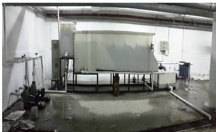
Name of Client: Eva Mall Location: Vadodara Capacity of Plant: 100 KLD STP Status : Active / Running
