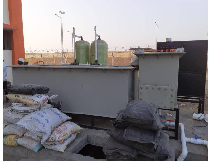
Name of Client: Camlin Life Science Ltd Location: Dahej SEZ, Dist.Bharuch Capacity of Plant: 40 KLD STP Status : Active / Running
