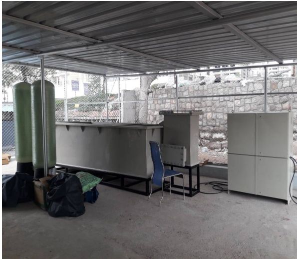
Name of Client: Enmedia Location: Hyderabad Capacity of Plant: 30 KLD STP Status : Active / Running
